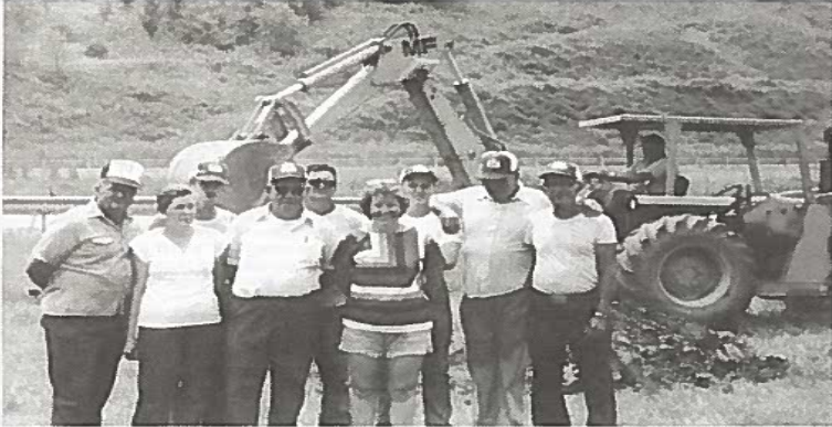
BUCKHANNON, WV — Surrounded by huge power shovel are members of Upshaw County REACT Team C117. Group saw first dirt moved for new headquarters building they had planned last summer. It will serve as a combination information center, emergency base and headquarters and will include a snack bar and two restrooms. It was built by volunteers and will be staffed for at least 16 hours a day and on holidays and Sundays as well according to Team President Burl Hewitt.
