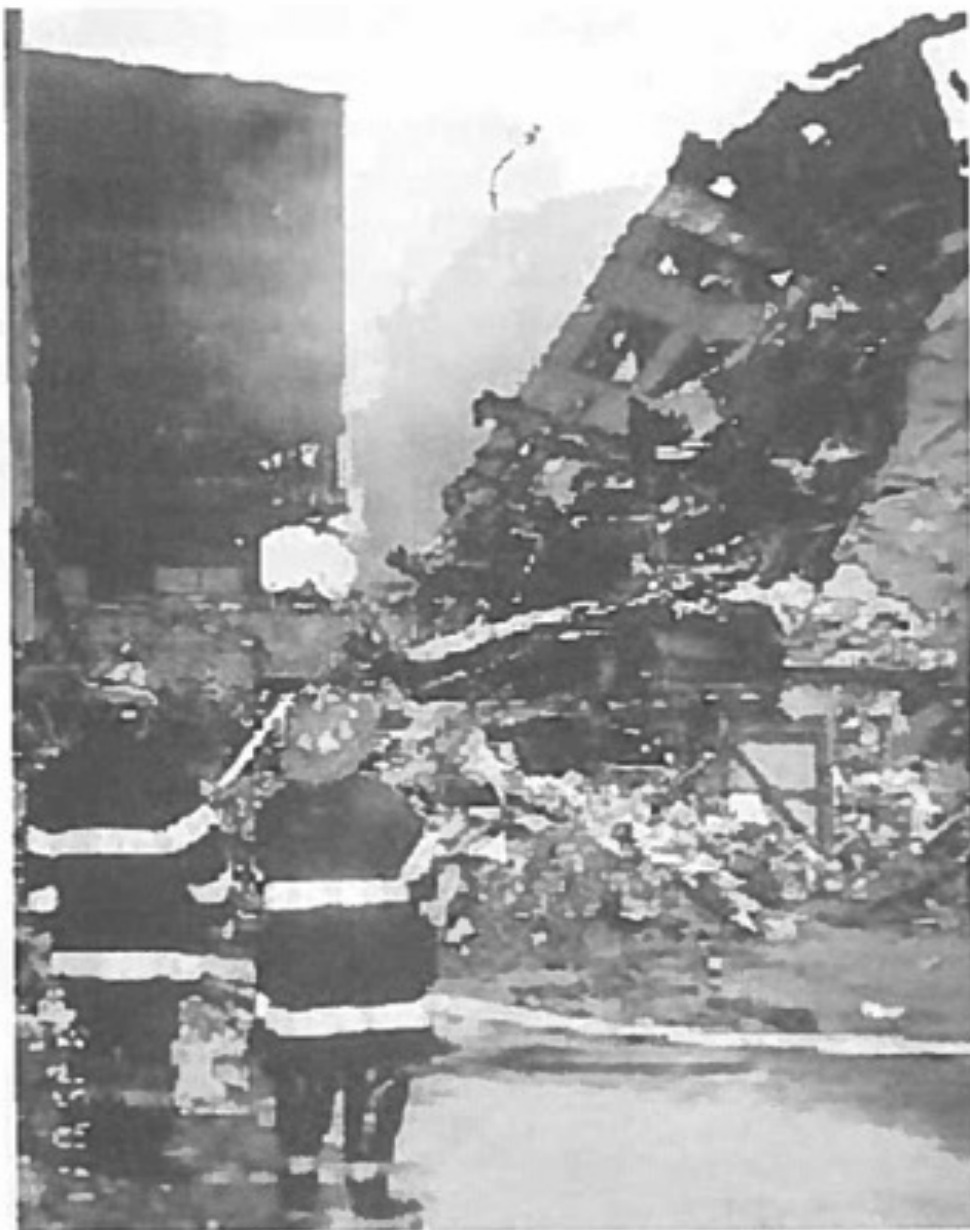
New York City firefighters at the World Trade Center site, a few days after September 11. (Photo: Clark Bortree.)
