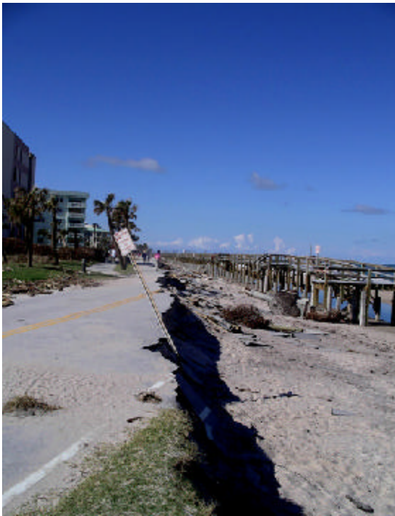
Hurricane Jeanne left this “road to nowhere” in Vero Beach, Florida. The condos at left have been condemned. The seashore is several miles to the right. (Photo: Linda Konrad)
