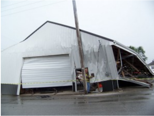
Francesville Fire Station Two sustained damage due to a tornado
