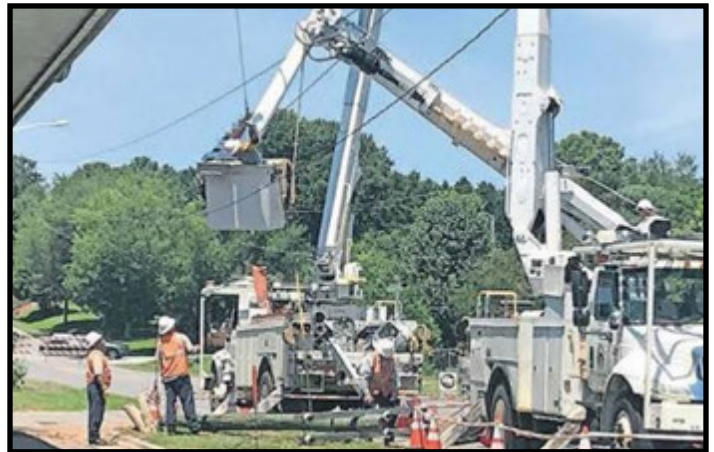
Crew in Shelby, NC work to repair damage done in a vehicle crash that claimed one life.
