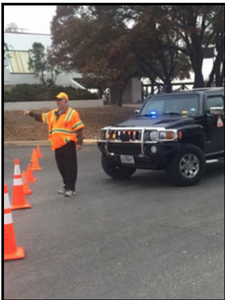
Member Donnie Hall assists with traffic while a gas leak is repaired in January
