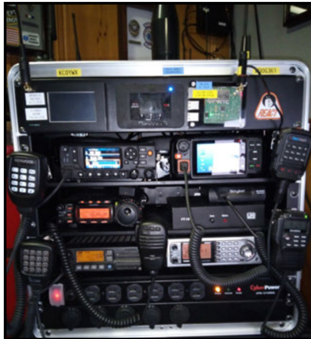
SE Colorado's Podcom box
